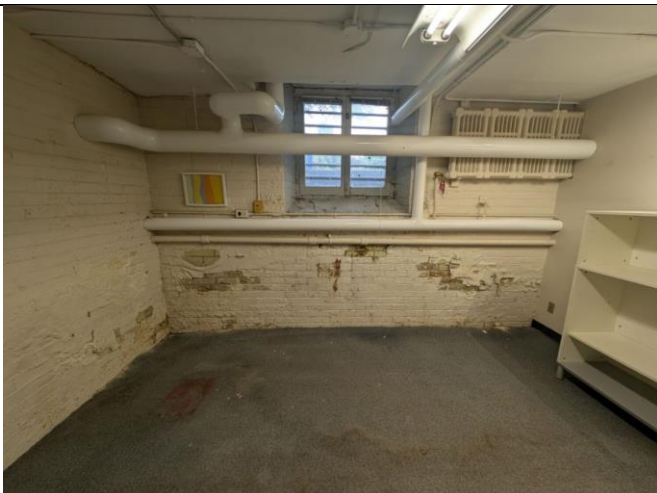
Photo 1: Basement, Room 10 Efflorescence observed along the perimeter of the brick wall.
