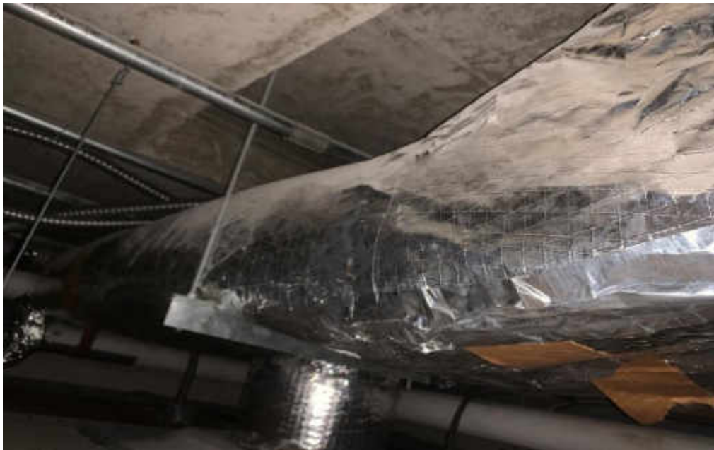
V0000, (None) Duct, Fibreglass insulated duct jacketed with foil, Corridor and Reception Area (Location #: 709)
