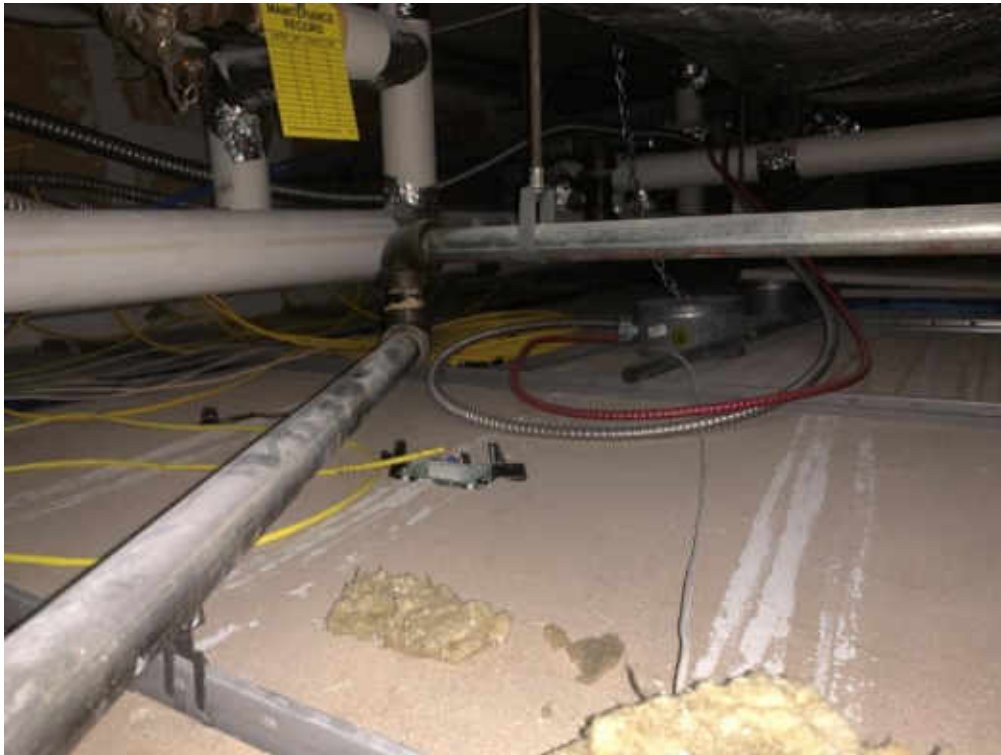
V0000 (None), Piping, Uninsulated pipes, Corridor and Reception Area (Location #: 709)
