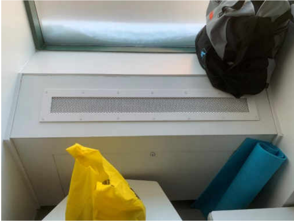
V0000, (None), Mechanical, Uninsulated Fan Unit, Room 7A26 (Location #: 708).
