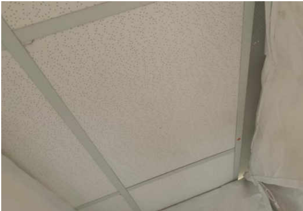
V0000, (None), Ceiling, 24"x48" acoustic ceiling tiles with pinholes, Corridor and Reception Area (Location #: 709)
