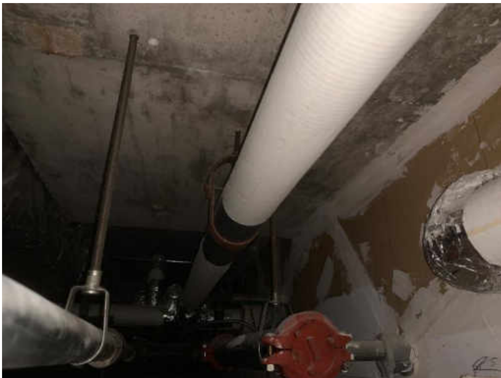
V0000 (None), Piping, Fibreglass insulated pipe jacketed with paper, Corridor and Reception Area (Location #: 709)
