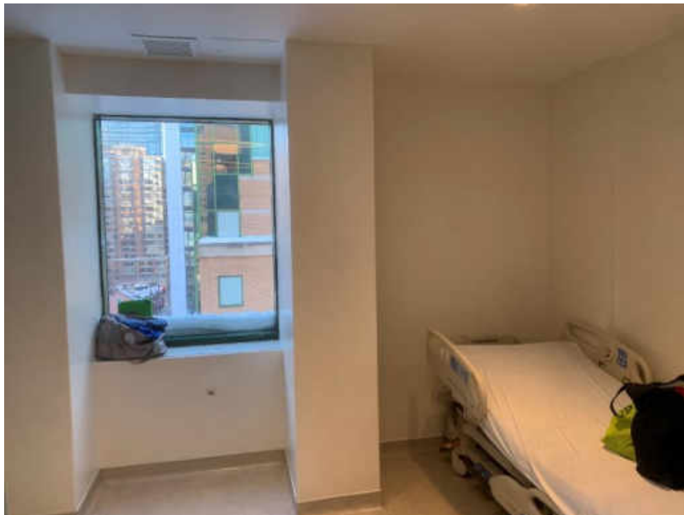
V0022, (Lead, None), White paint on drywall wall, Room 7A29 (Location #: 710)
